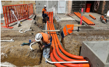
Margaret Street Pump Station
